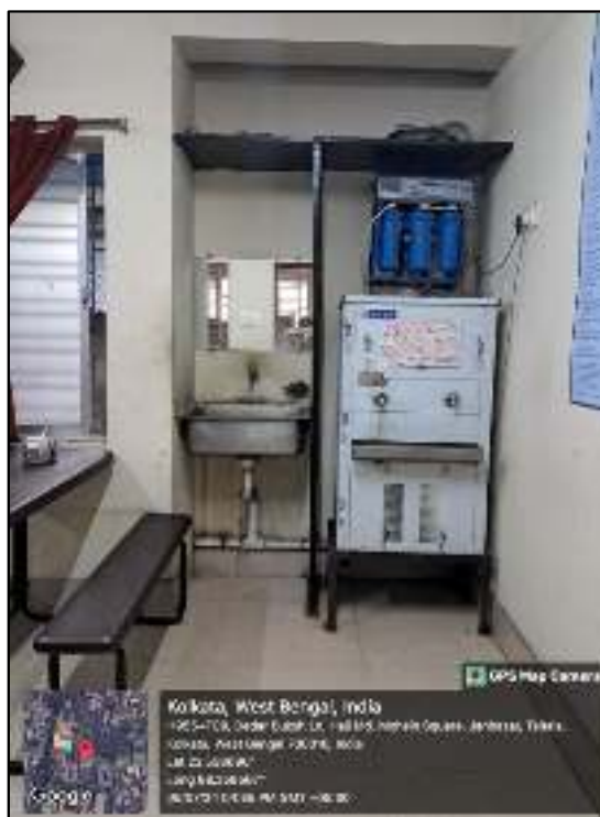
DRINKING WATER-CUM-COOLER FACILITIES
