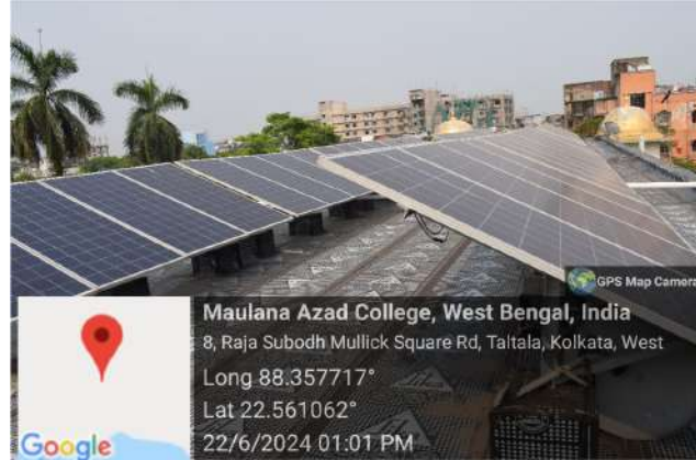
Rooftop Solar Panel
